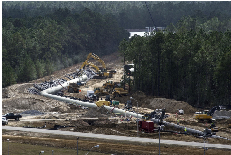
A high-pressure water pipeline being installed at NASA's Stennis Space Center. Credit: NASA.
